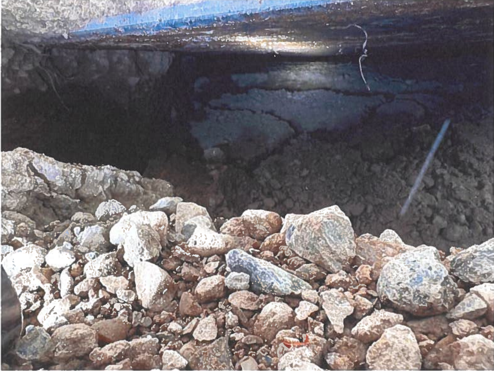
PHOTO 2 – SUBGRADE EROSION UNDERNEATH STEEL PLATE
